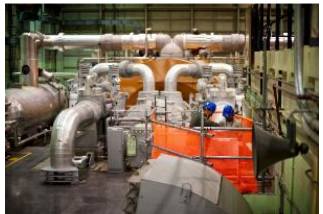
Contractors perform some pre shutdown maintenance in the generator room. The Xcel Energy Prairie Island Nuclear Plant north of Red Wing is looking to boost electrical output at the plant. Tuesday, October 9, 2012
